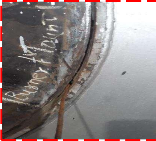
Crack found after MPI
